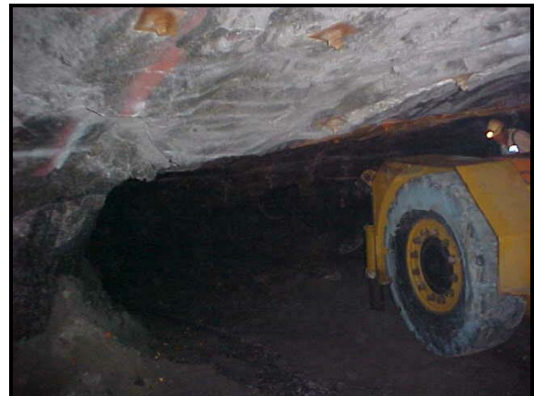
Pillar edge showing hourglass fracturing
