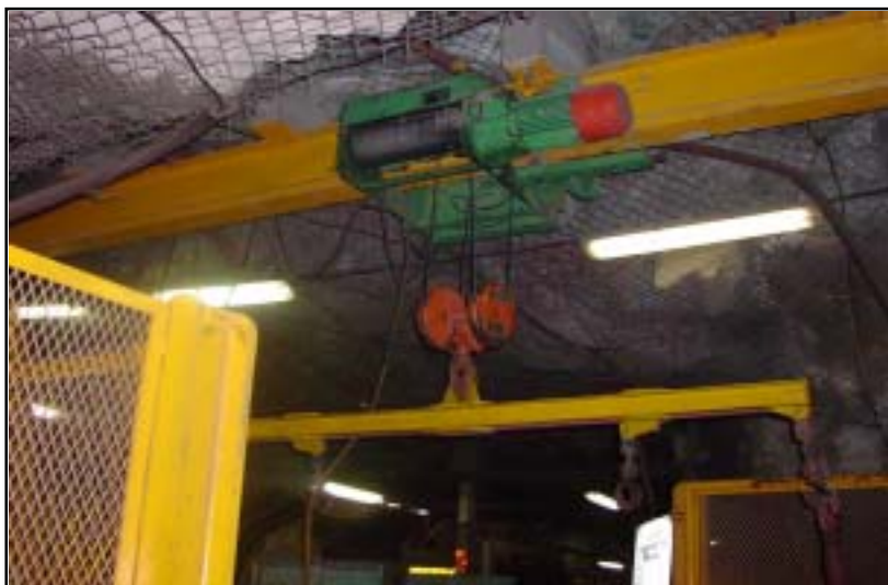
View of overhead crane
