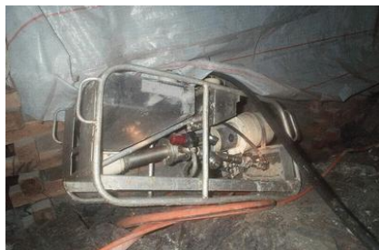
Figure 36. ACE porcupine pump in use from 1988 to 1992
