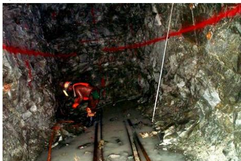
Fig 34. Blast with ANFO and CFIC showing large number of sockets and poor condition of sidewall (base case).
