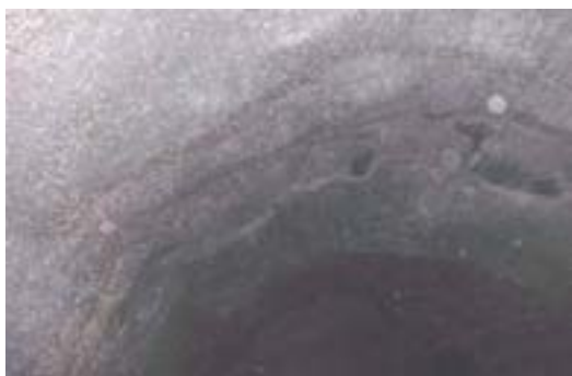
Figure 8 – showing general view of condition of supported silo
