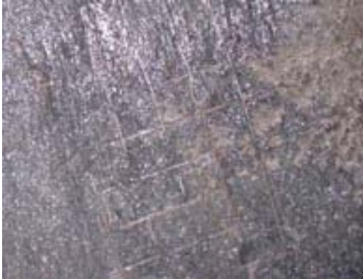
Figure 10 – showing shotcrete eroded to partially reveal weld mesh
