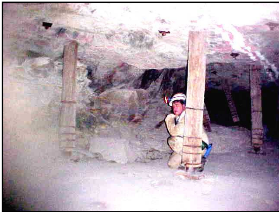
Photo 2 Scaling of the updip crush pillar
