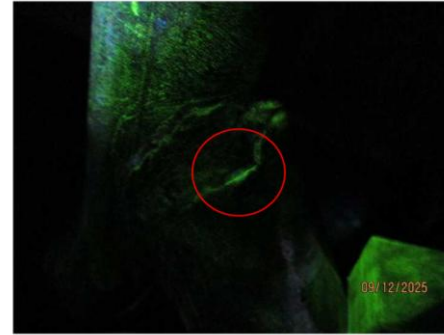
Fig 17: Chairlift No: 112 Crack like indications noted.
