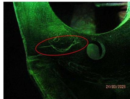
Fig 15: Chairlift No: SI/17 Crack like indications noted.
