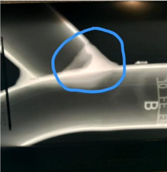
Pipe cut short – filled with welding
